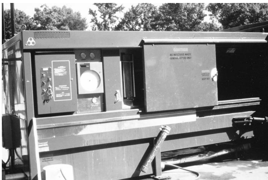
Fig. 8.8 On-site steam autoclave
